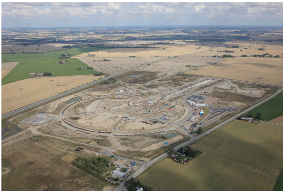
ESS construction status in Oct. 2015 with growing parts of cast accelerator tunnel and started piling of target station.
